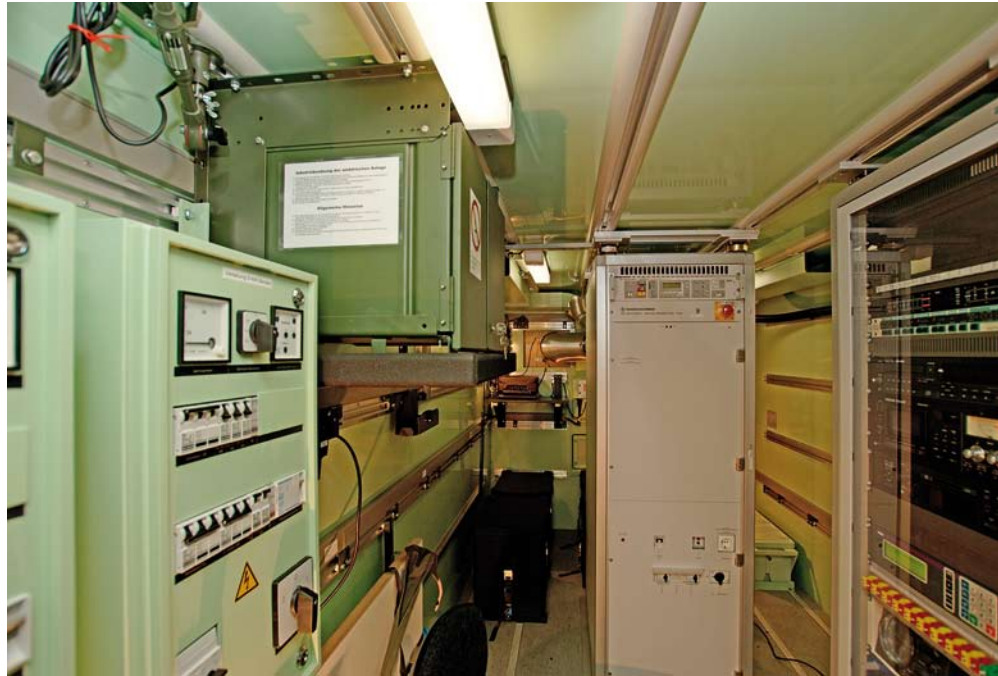
FIG 2 Shelter with power distribution (left), VHF FM transmitter (center) and resilience audio supply unit (right).
